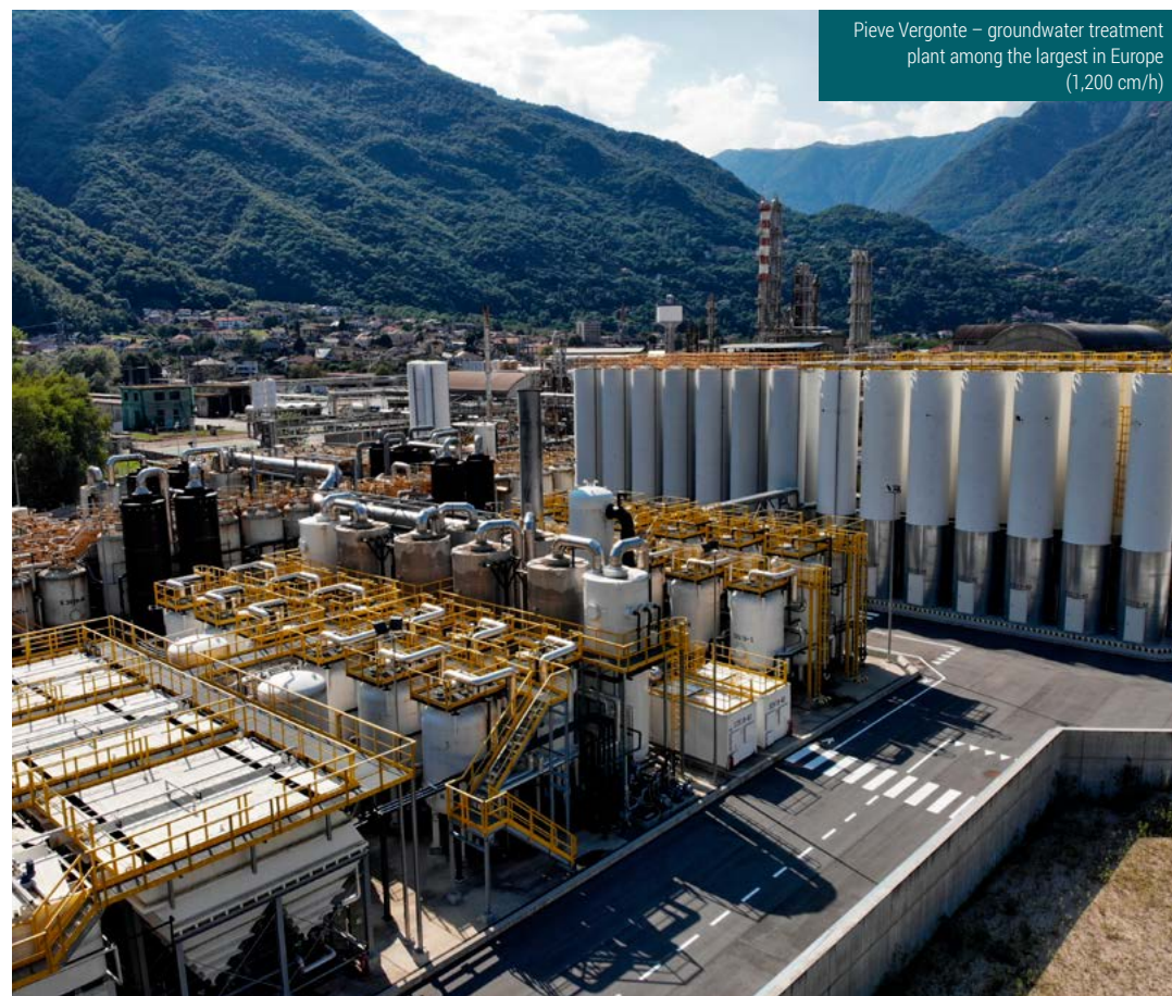
Reverse osmosis plant
